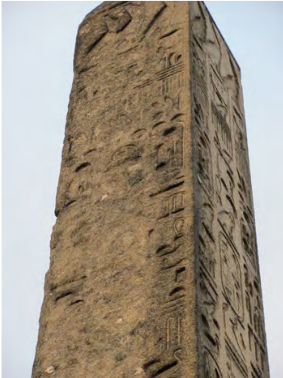
Close-up of text on the obelisk, which has been severely eroded from exposure to the elements. (Photo: Richard Paschal and Dorothy McCarthy)
